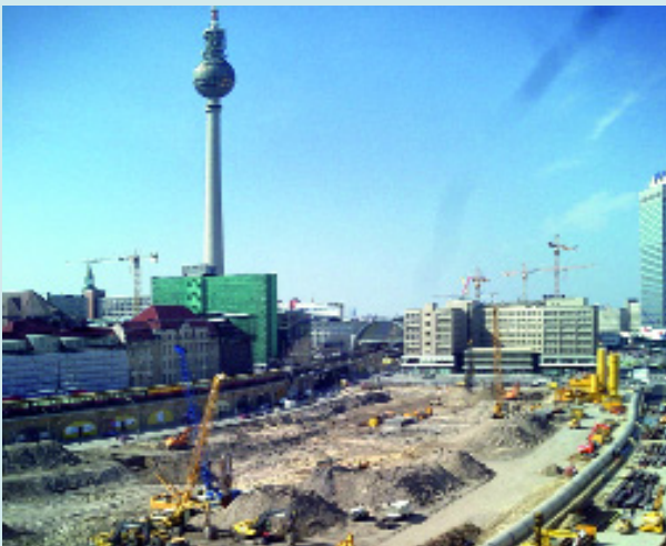
Temporary sewer bypass DN 2200 at Alexanderplatz, Berlin. Reproduced with kind permission of beton & rohrbau C.-F. Thymian GmbH & Co KG, Berlin
