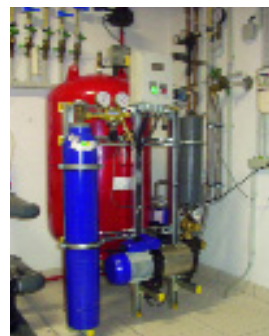
Underground water purification system UWEMAoxygen.
